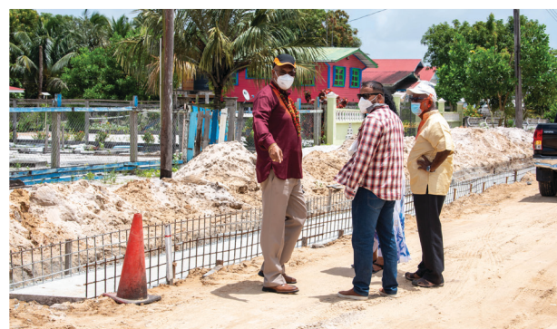
Minister of Public Works, Bishop Juan Edghill MP inspecting the Lima Sands access road
